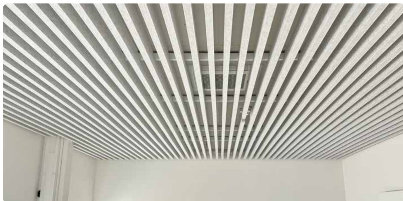
Quick grid ceiling installation with a clean, linear appearance and an integrated air conditioning unit behind, as well as a recessed smoke detector.
